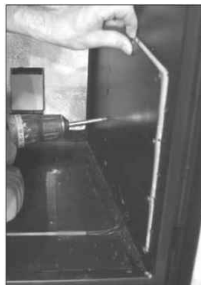
Figure 57: Removing Access Cover.
