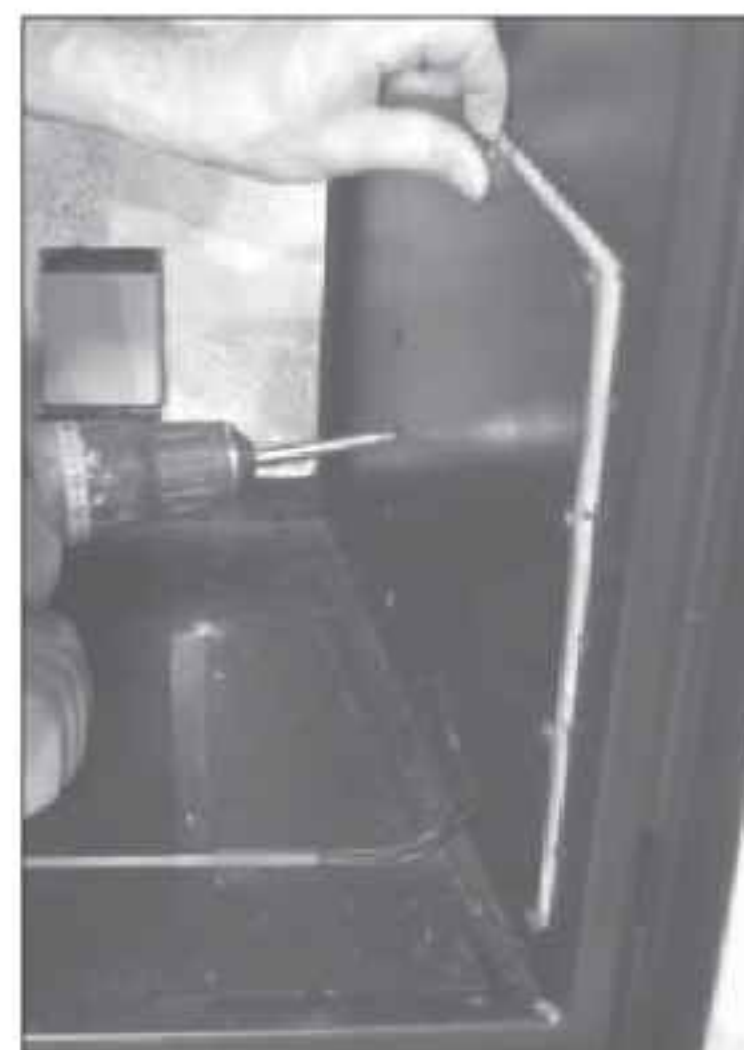
Figure 57: Removing Access Cover.
