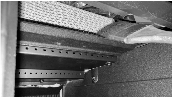
Fig. 6.2. Use a soft brush to clean the combustor.
