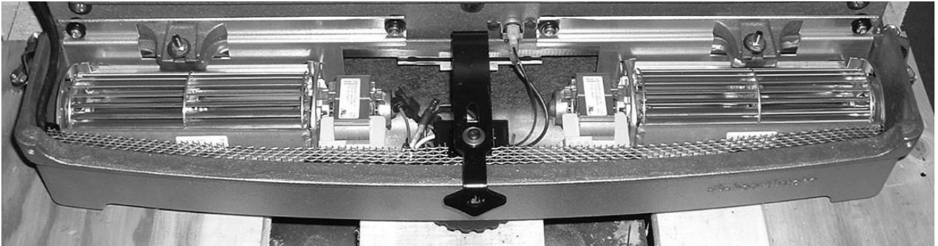
Photo 30 – Blower System (Ash Lip Cover Removed)
