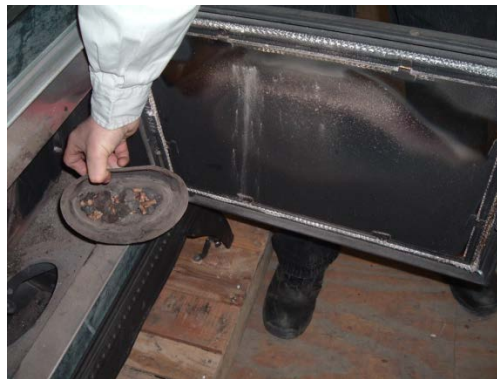
Burn pot has buildup. Blackened glass indicates air restriction from blockage or poor draft.
