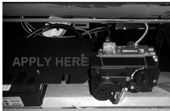
Figure 15 – Valve Warning Label Location
