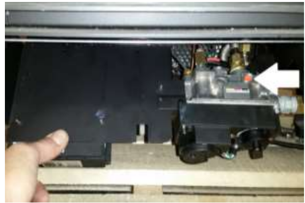
Figure 12 – Low Pressure Orifice Access, Valve System Tilted Down.
