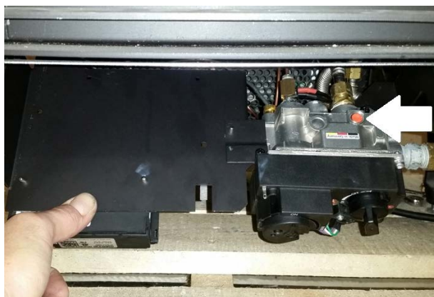
Figure 7 – Low Pressure Orifice Access, Valve System Tilted Down.
