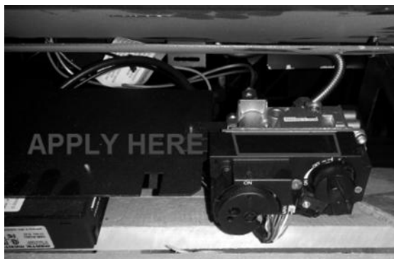
Figure 15 – Valve Warning Label Location
